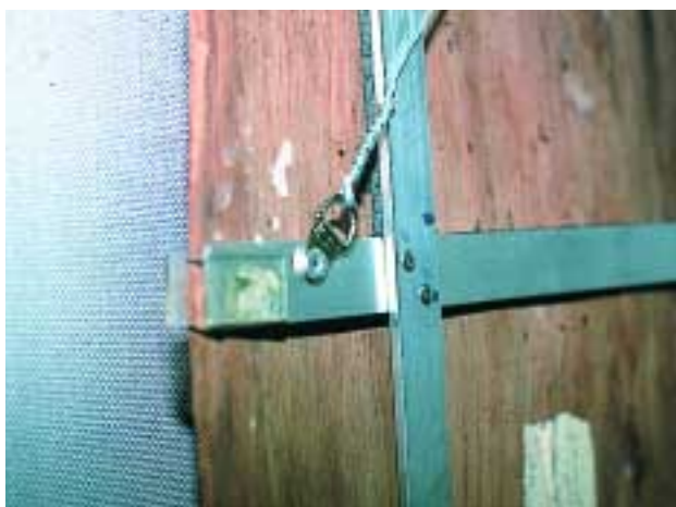
Mount system with D-rings and polycarbonate clips in place.
